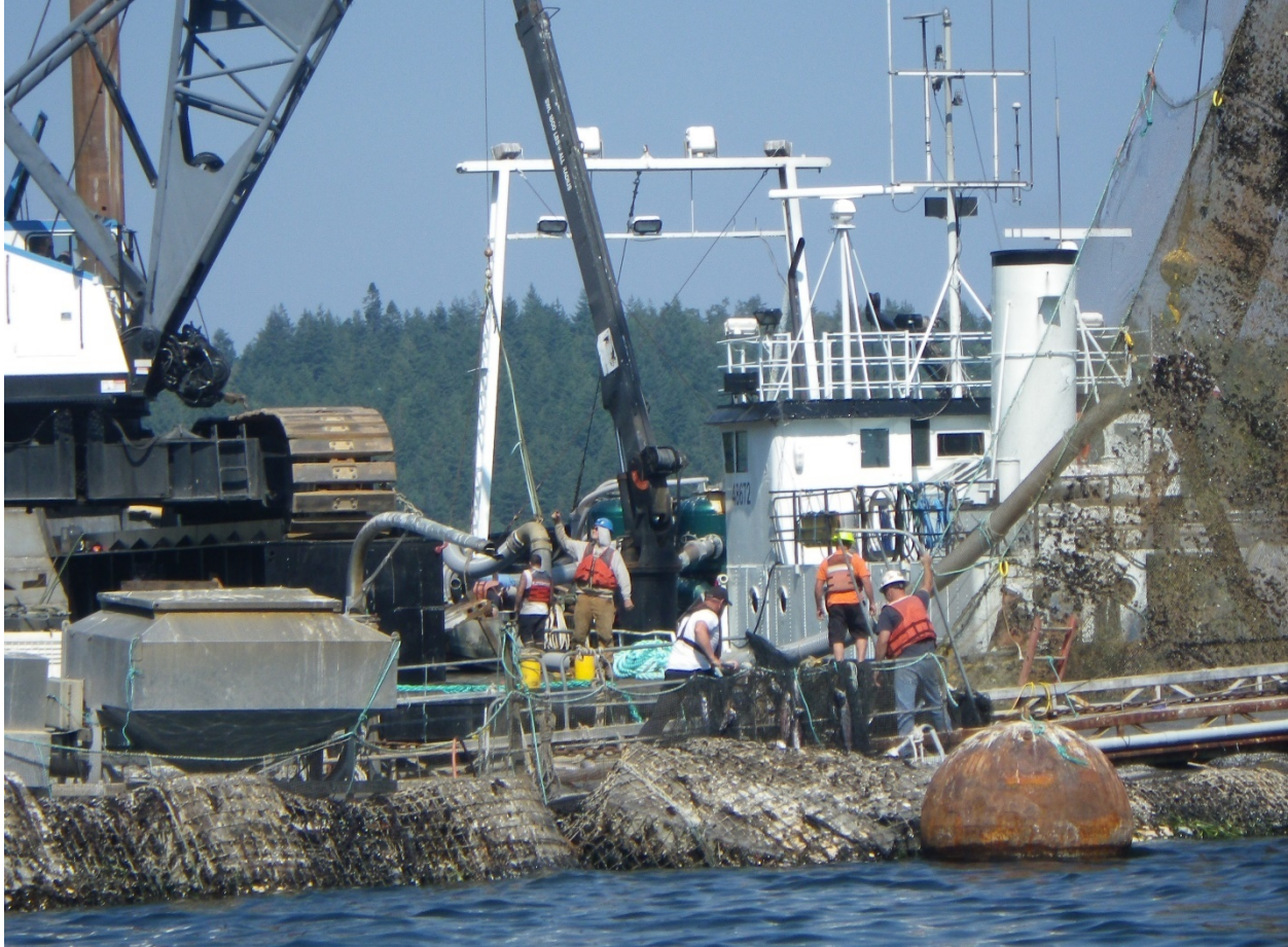
Figure 30. Image possibly showing preparation for extraction not using divers at 2:24 p.m. on August 29. Note gray 12-inch hose lying on deck of crane barge and elevated toward the stern of HARVESTOR (at right), apparently stretching from the vacuum pump.
