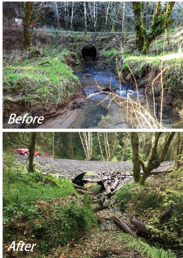
Figure 20: Fish-barrier Removal on an Unnamed Tributary to the Chehalis River. This project replaced one 96” culvert in a highly incised channel with a 20’7” wide by 13’2” tall multi-plate pipe arch. Large woody debris was placed in the downstream channel to improve fish habitat. A total of five miles of salmon and trout habitat were opened up as a result of this project. Photos courtesy of Jerry Mizar and Will Hoskins.
