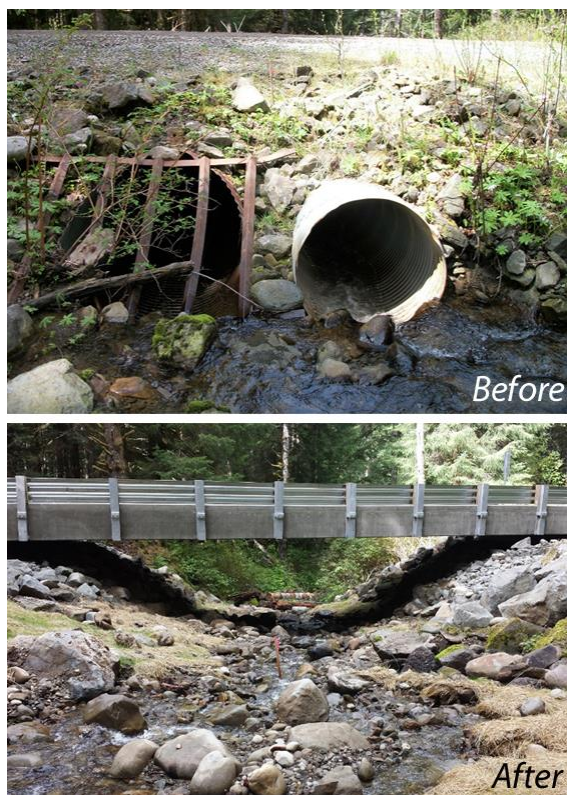
Figure 8: Fish Passage on an Unnamed Tributary of the Hoh River. DNR replaced a 60-inch culvert and debris rack and an adjacent 42-inch culvert with a 60-foot concrete bridge, opening up 1,500 feet of fish habitat. Photos courtesy of Candace Montoya.
