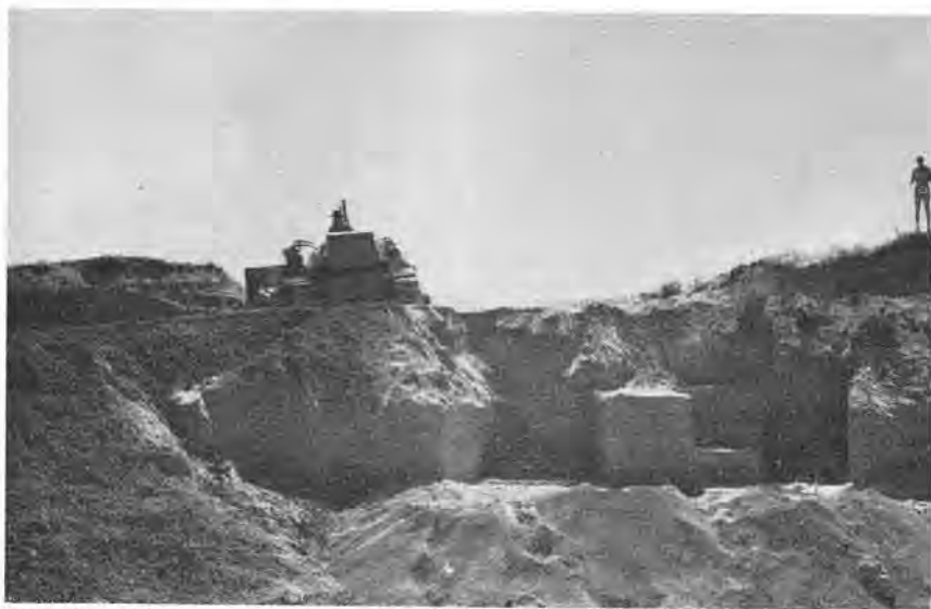
FIGURE 9.—Bulldozer at work removing sterile overburden from culture-bearing stratum. The overburden was removed to the level of the flat-topped pedestal in right-center foreground. View facing east.
