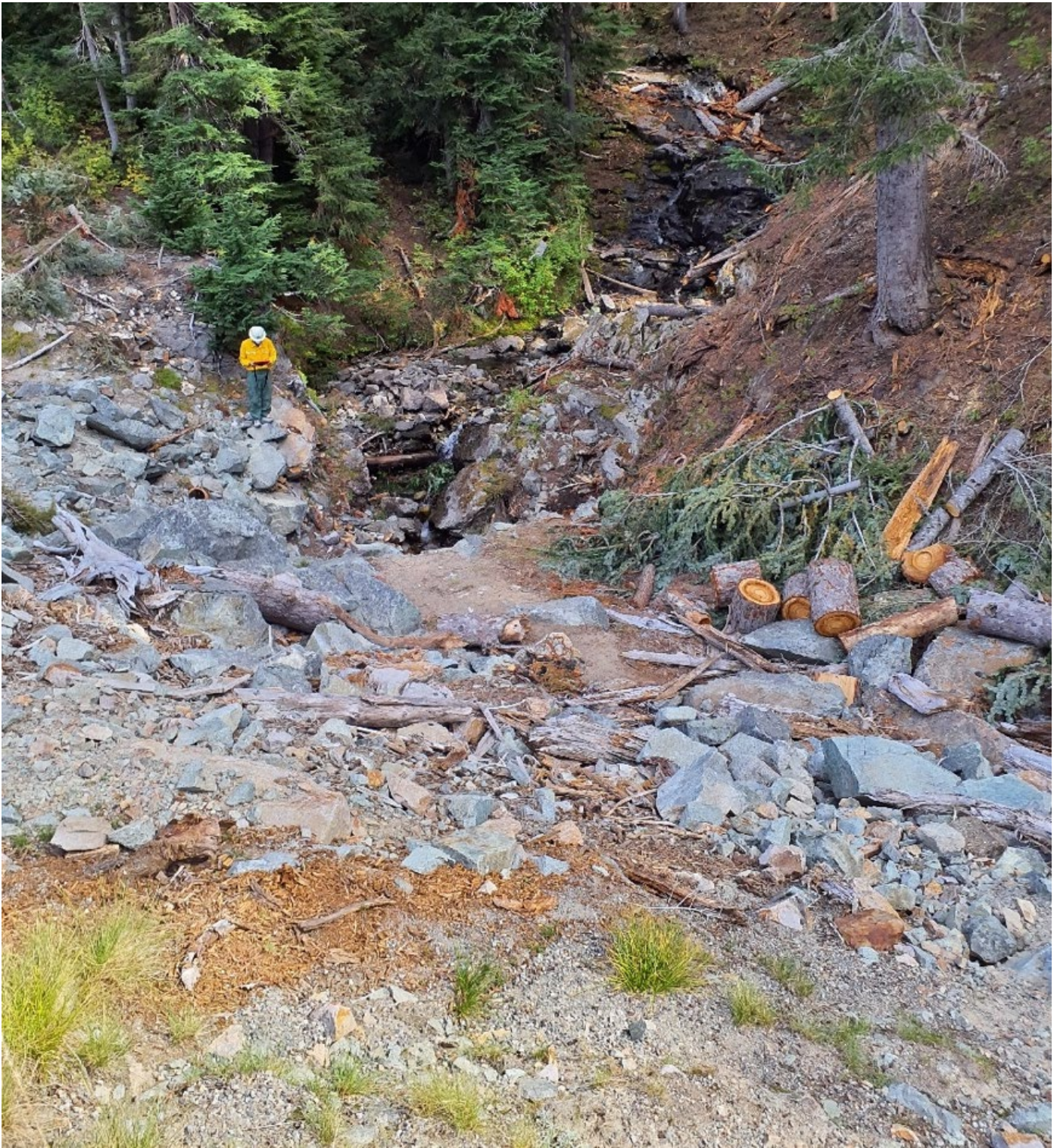
Figure 3. Stream channel conditions adjacent to State Route 20, looking east at culvert inlet side, for the Blue Lake Fire.
