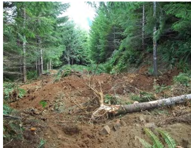
Example of Recently Abandoned DNR Forest Road. Photo: DNR
