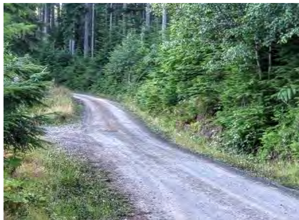
Standard Best Management Practices to Minimize Erosion Include Placing Crushed Surface Rock on Roads. Photo: DNR
