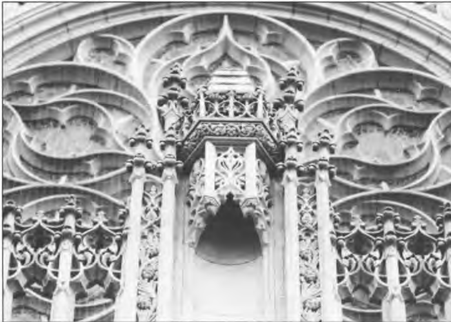
Figure 7. An example of Walker-Wilkeson sandstone on the Cathedral of Saint John the Evangelist in Spokane (1926–1954). This carved detail is below the western rose window (covered by a mesh that prevents birds from nesting on the stone). The building's exterior is made of the sandstone, and the interior is made of Indiana limestone and Boise sandstone.
