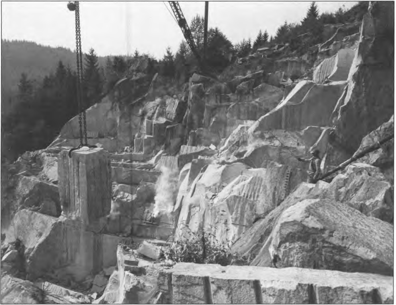
Figure 9. Lifting a 35-ton block (about 6 ft x 6 ft x 12 ft) of Walker-Wilkeson sandstone out of the quarry after dimensional blasting. Signaler on the right is steadying a line (above photo frame). Steam rises from a jackhammer drilling to prepare for blasting. Bedding in this quarry dips about 53 degrees, too steep for using channeling equipment. 1950s photo courtesy of Robert Walker, Jr.
