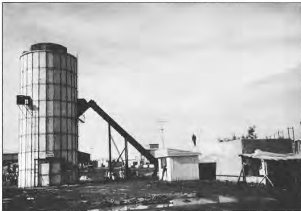
Figure 14. A newly constructed wood waste burner in Chile, the first of many that Olivine Corp. of Bellingham anticipates selling in South America. The burner runs continuously to eliminate sawmill waste from present and past production of extensive planted Radiata pine (Monterey pine hybrid) forests. The burner is made of refractory (heat resistant) olivine bonded in cement. The olivine is produced in the Cascade Range southwest of Mount Baker.
