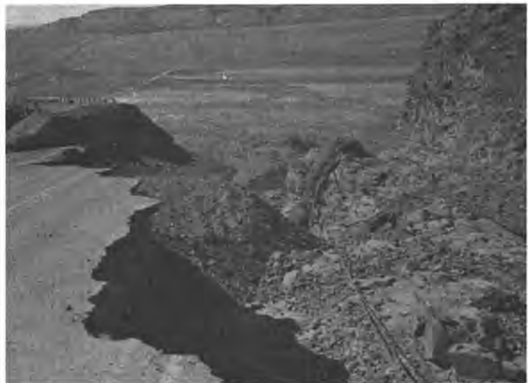
FIGURE 2.—Flash-flood damage to westbound lane, gabion-lined drainage channel, and wash-out of all three lanes and 50-foot-deep fill. East wall of Moses Coulee, looking southwest.
