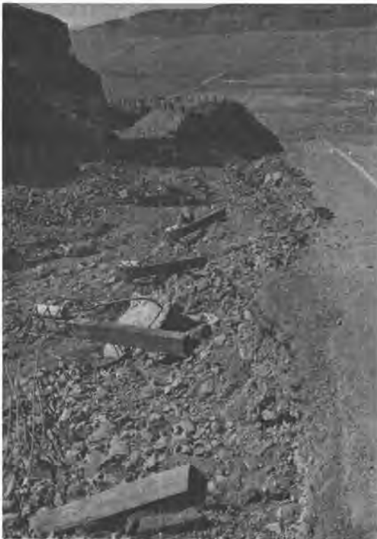
FIGURE 1.—Flash-flood damage to eastbound lanes, and washout of pavement and 50-foot-deep fill, U.S. Route 2. Looking southwest into Moses Coulee
