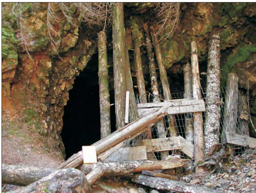
Figure 7. Opening to Big stope. Notebook (8½ x 11 inches) for scale. View to the west.
