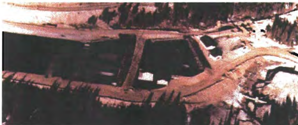
Figure 10. Aerial view of the construction of the West End project heap-leach pads and ponds at the Stibnite mine, Idaho, in 1982. Pads consist of asphalt set on glacial sediments. These asphalt-lined pads are unloaded after heap neutralization and then reused. (Photo provided by Ray Lasmanis, Washington Department of Natural Resources.)
