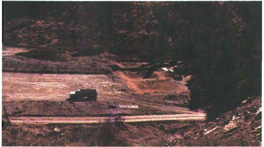
Figure 15a. Initial construction of a heap-leach pad and pregnant and barren solution ponds in 1984 at the Minnie mine (Fig. 14). Each pond could hold about 80,000 gallons. Ponds used a double geomembrane liner system with leak detection placed on a compacted soil base. (Photo by Rod Lentz, U.S. Forest Service, Okanogan National Forest.)
