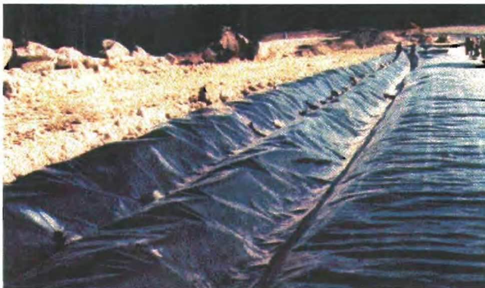
Figure 6. Preparation of a heap-leach pad and liner at the Coeur Thunder mine in central Idaho in 1985. A sheet of impermeable geomembrane is laid down on a slightly inclined surface of compacted low-permeability glacial till, and the ore is then stacked on top of the sheet. Lined ditches contain and collect solutions. (Photo courtesy of Bruce Schuld, Idaho Department of Environmental Quality.)
