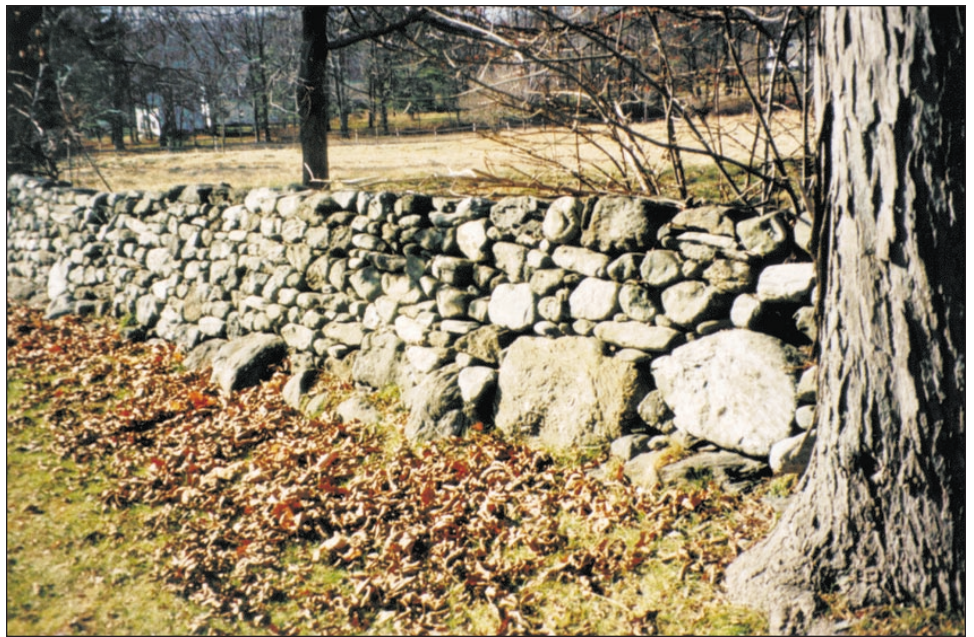
Figure 2. A dry-stacked stone wall in Connecticut. Notice the rounded edges of the stones, the wide base, and the placement of the largest stones at the bottom of the wall. Photo by Eric Gerstel.
