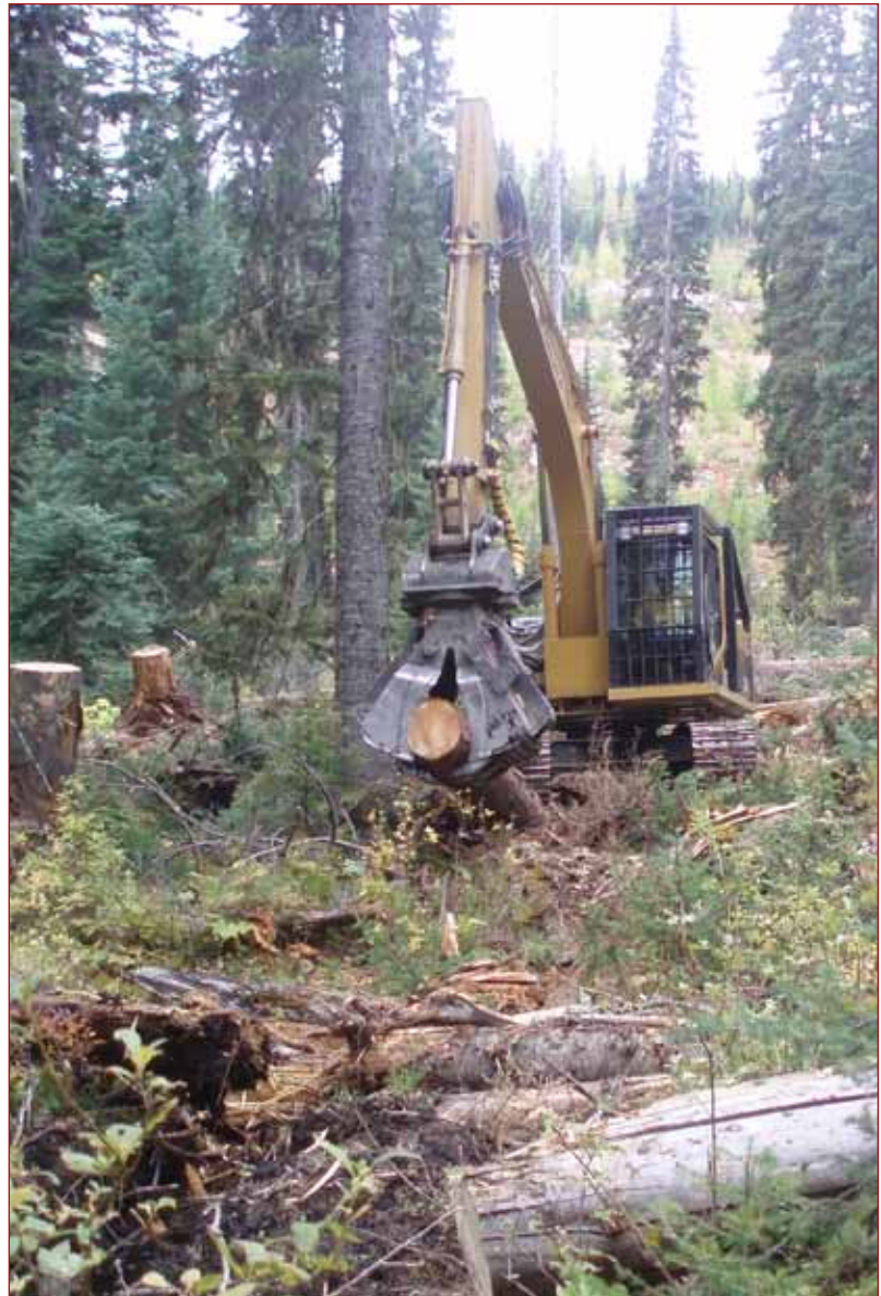
Minimal impact in riparian area achieved by laying logs and brush down for tracking over.
