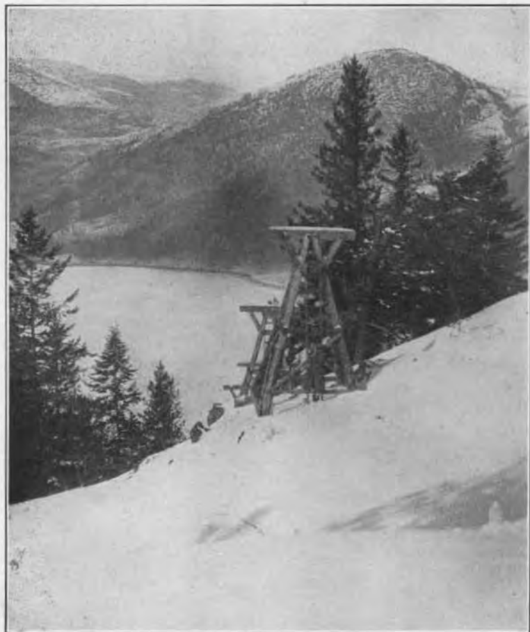
Looking down the tramway of the Copper World Extension Mine, from point near tension station. Palmer Lake below.
