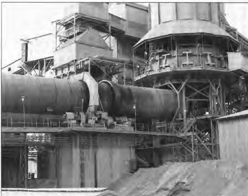
Figure 4. Dolomite ore reaches the smelter on a conveyor belt and the smelting process begins when it passes through the rotary kiln (center to left center) on its way to one of six furnaces. In this stage of the operation, carbon dioxide is driven off to produce a lime product called dolime.
