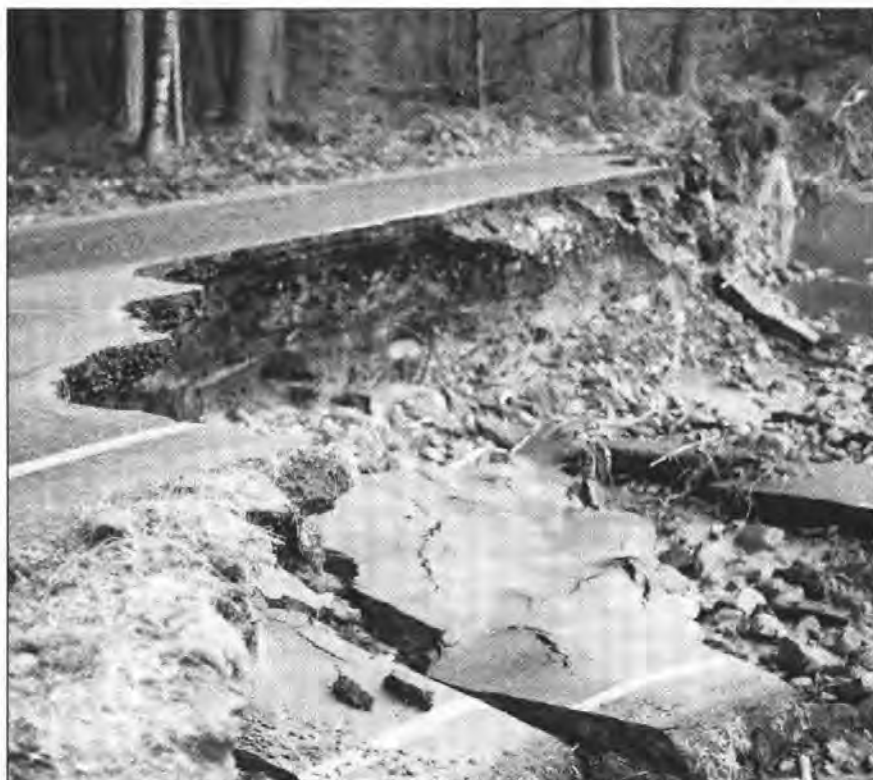
Figure 1. A major washout on the Cispus River Road (FR 23).
