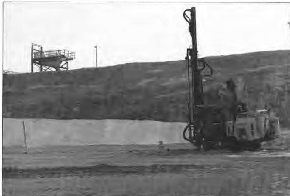
Figure 3. Dolomite at Northwest Alloys dolomite mine at Addy is drilled prior to blasting. After blasting and transport to a crusher, golf-ball-size ore material is separated out and sent to the smelter (cover photo) to produce magnesium metal.
