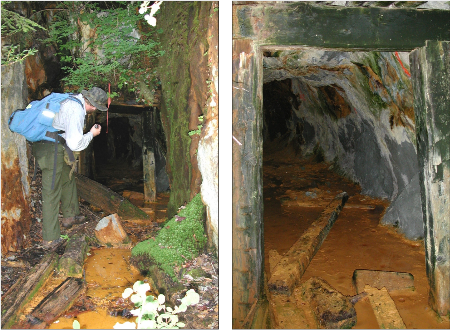
Figure 9. Outside main adit at the Lockwood Pyrite mine. Analysis of discolored mine drainage (foreground of photo on left) confirmed acid mine drainage and dissolved metals. View inside adit portal (photo on right) shows massive sulfide deposit on adit walls and acid mine drainage on adit floor.
