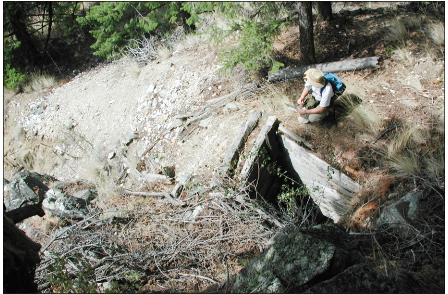
Figure 16. Open shaft with timbered collar at the John Judge mine. This shaft is reported to be 182 feet deep. Litter and debris are visible at ~40 feet; this may not be the actual bottom. Open cut (to left) leads up to a collapsed adit intersecting the shaft.
