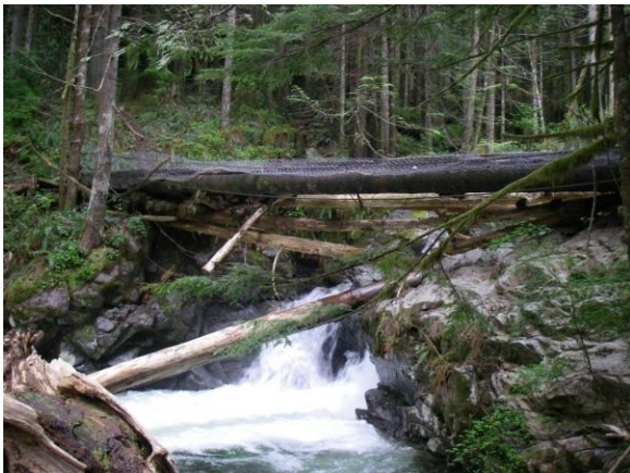
User-built structures such as this log bridge with chicken wire nailed to the top present risks to public safety and potential liability issues for DNR.
