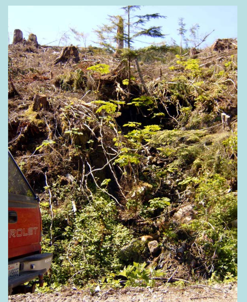
Seeps and sapping occur in road cuts along earthflows.
