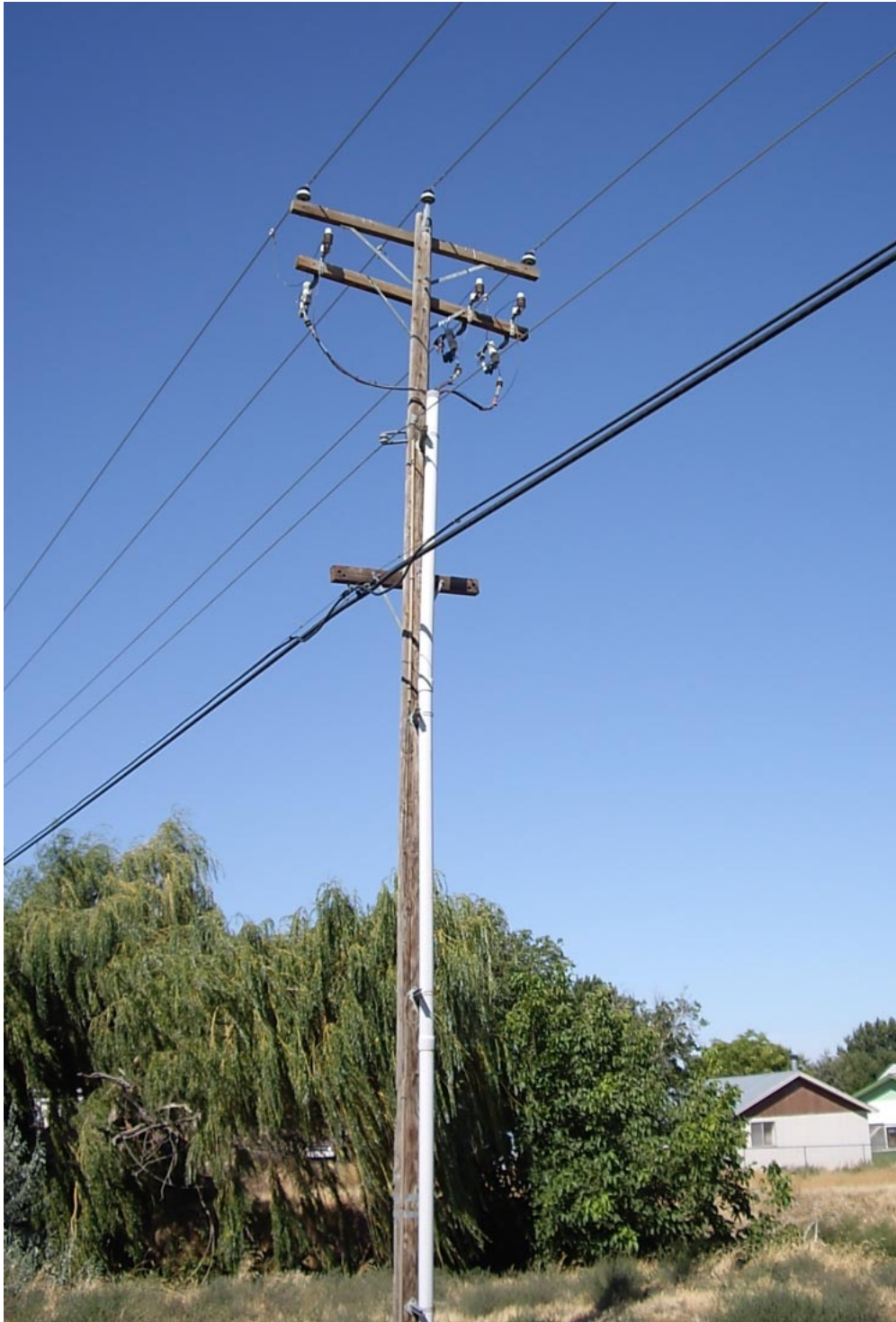
Telephone poles made from trees can last 75 to 100 years. Steve Thorne/ Benton (County) PUD Photo
