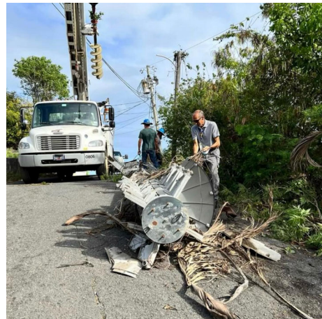
Tsunami reinstallation by Deputy Director of Logistics, Stephen Deblasio, the project lead.
