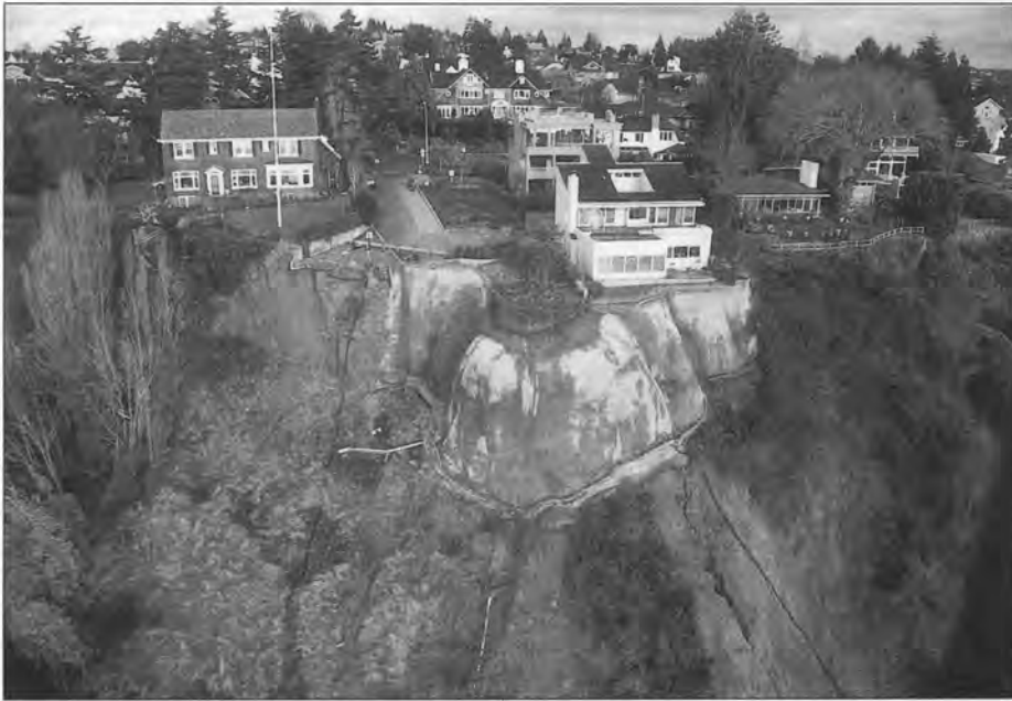
Figure 27. Shotcrete, shown here, has been used (not always successfully) to prevent surface erosion and headward migration of the bluff edge. The drainage must be directed away from the base of the cover so that the shotcrete will not be undermined by surface erosion. The drainage must also be continually maintained in order to be effective. In this location, there is extensive erosion occurring at the base of the shotcrete cover. If the material behind it is washed away, the shotcrete will fail, as seen in Figure 11.
