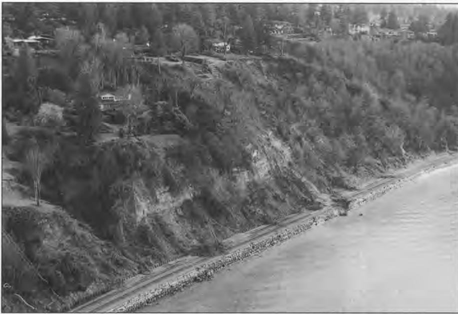
Figure 22. This view to the south shows a few of the many recent debris flows along the section of the railroad tracks north of Carkeek Park (Fig. 1). Exposed in the lower half of the bluff face are dense water-perching clays and clayey silts, which have not moved at this location. These maintain a steep bluff face that is often wet due to ground water seeping from the contact with the overlying sand. The weaker overlying sands have a much gentler slope. In the upper middle part of the photo, one can see the headscarps of older, vegetated landslides that have progressed farther back into the highlands. These features illustrate the continuing differential retreat rates of the upper and lower portions of the bluff (see Fig. 21C). The home in the left center of the photo sits in one of these landslide scars. This view shows the bulkhead that protects the toe of the slope from wave erosion (discussed in Fig. 12).
