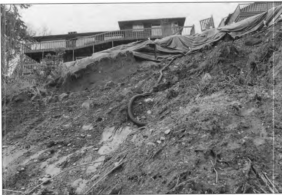
Figure 18. This shoreline home between the Hood Canal Bridge and Port Ludlow lost its front yard during the December/January rainstorms and snowmelt. Bedrock exposed on the beach below the bluff shown in this photo was resistant to wave erosion. However, the glacially polished bedrock perched ground water in the gravelly sand above the steeply sloping contact here. Runoff from rapid snowmelt was apparently funneled down the driveway from upslope development. The area to the left of this landslide (out of view) was probably buttressed by a large maple stump kept alive by sprouts. (The area still farther left also failed.) Glacially compacted silts or bedrock form a barrier to roots and ground water. Where this condition exists in the Puget Lowland, shallow debris avalanches can be common. The overlying permeable saturated soil cannot be anchored to the substrate by the weak toehold of the roots of trees and other vegetation.
