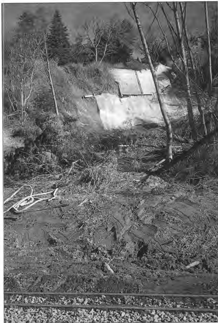
Figure 29. A resourceful homeowner in the area north of Carkeek Park, along the BNSF Railroad, used metal roofing material to cover the upper portion of the slope below his house. However, the lower part of the slope failed as a debris flow onto the railroad tracks during the December/January storms, probably because energy from runoff water was not properly dissipated, thereby causing erosion below the roofing material. Subsequently the lower slope was covered with strips from large rolls of plastic sheeting. Placing the plastic required the use of technical climbing equipment by skilled workers seen here to the left of the sheeting.
