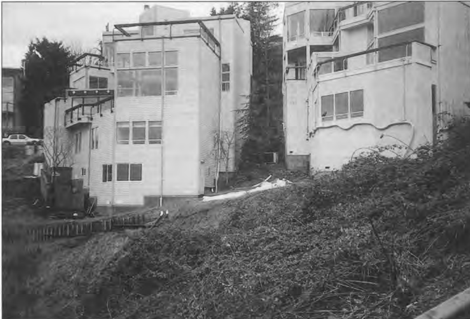
Figure 28. These two apartment buildings in the Duwamish Head area of West Seattle, just south of the intersection of Ferry Avenue and California Way SW shown in Figures 4 and 8, are built at the head of a small ravine on unconsolidated sand deposits. The February 1996 storm resulted in a shallow debris slide in that ravine. As a result, drainage from all the roofs and balconies is now collected in nonperforated pipes and directed away from the steep slope. This is called tightlining, and it is also effective along beach bluffs. There were no slides directly below these buildings as a result of the December/January storms.
