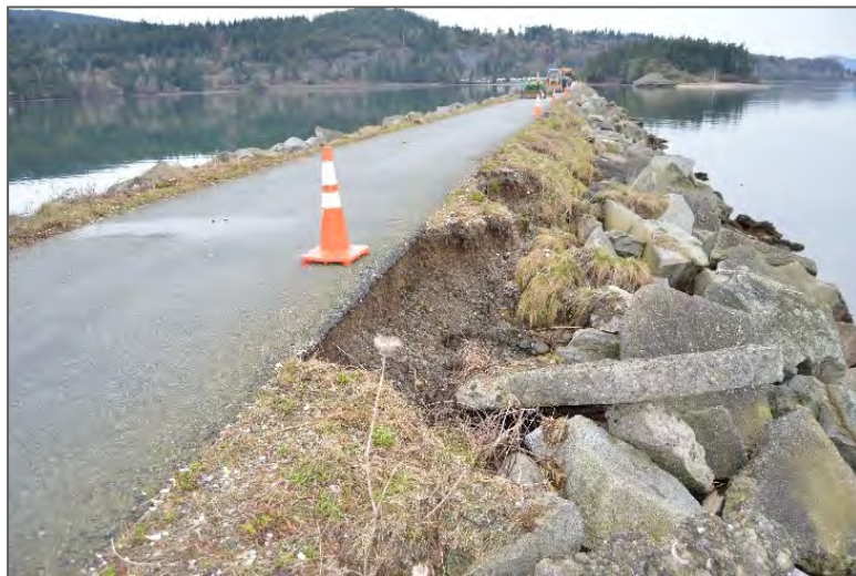
Figure 9: February, 2015 damage to the causeway revetment from storm surge (Photo: DNR).
