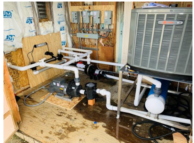
Fig 1. The pump room upgrades are complete. Two new pumps have been installed to pull water from the Puget Sound and to push water through the filtration system. The chiller, to the right, was installed inside the pump room alongside some major electrical upgrades.
